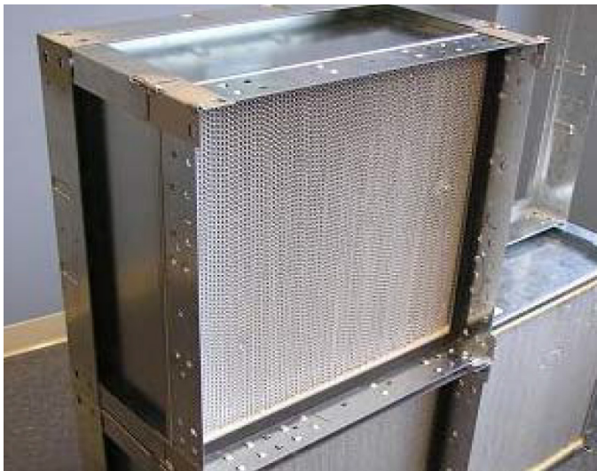
Figure 50: Properly Installed HEPA Filter
